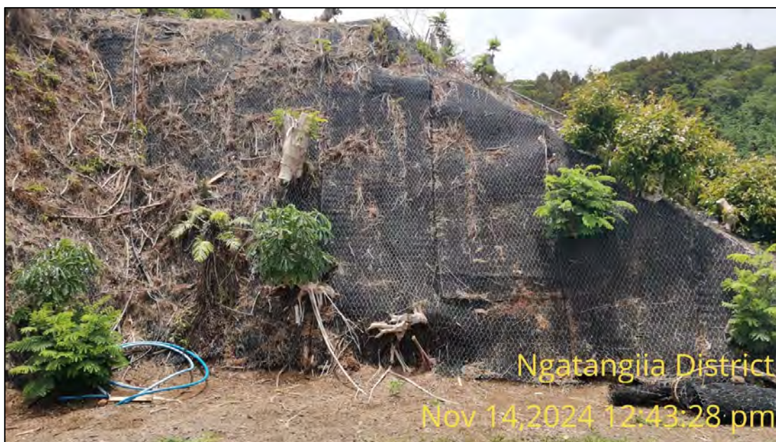
Figure 6: Geotextile matting reinforced with steel mesh, applied some 17 years ago along the adjacent property.
