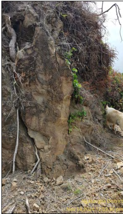
Figure 4: Observe dense soils and weathered volcanic rock, remnant of past excavation works, in this regard the 4m high cut face is adjacent to the existing water storage tanks. The earthworks was undertaken in 2010 and has remain in place without a retaining wall for over 14 years.
