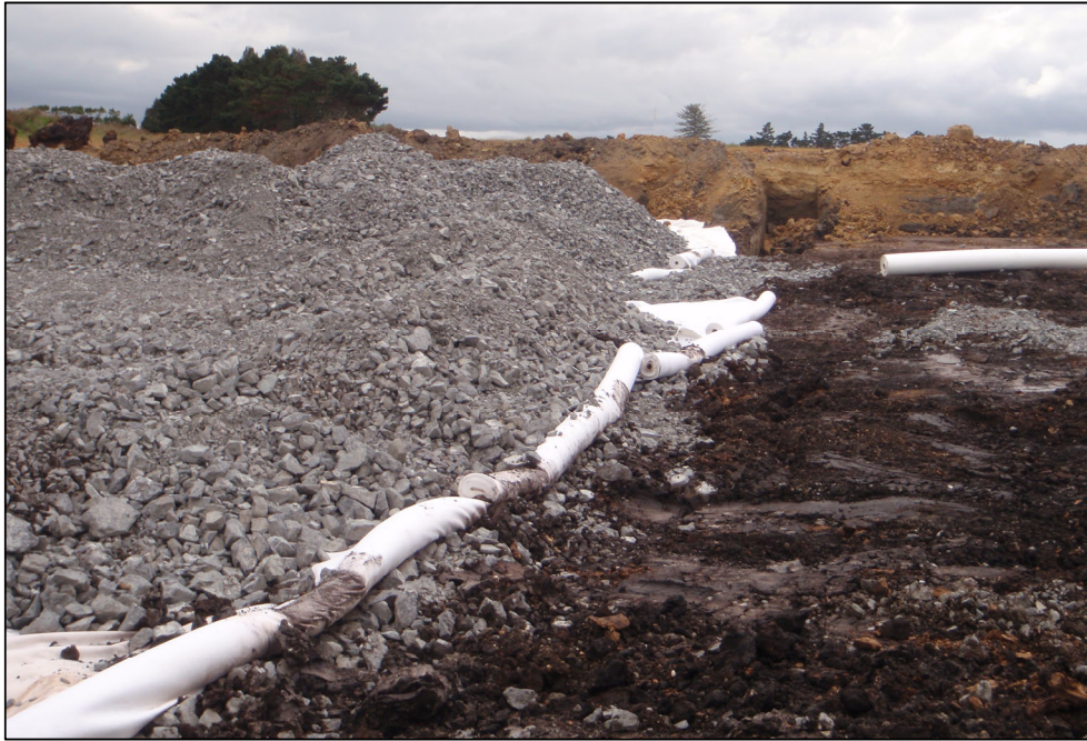
Figure 4: Geotech Fabric placed beneath granular fill over soft ground (image source: Cirtex GeoSynthetic Solutions)
