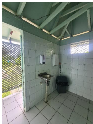
Public toilet opposite Police Station in need of an upgrade.
