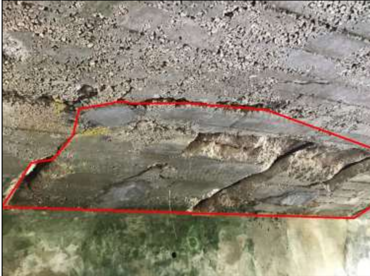
Figure 1 Extensive spalling of concrete arches including concrete cover (August 2021 Inspection)
